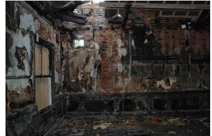
Current photograph illustrating fire damage to upper floor
