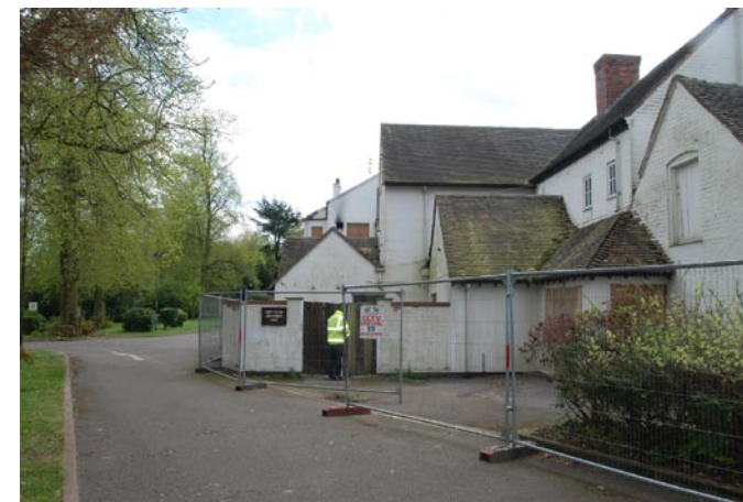
Two storey and single storey extensions added in 1990s. Constructed in rendered concrete blocks with trussed rafter and loose rafter roof construction - present poor image to Tamworth Road.
